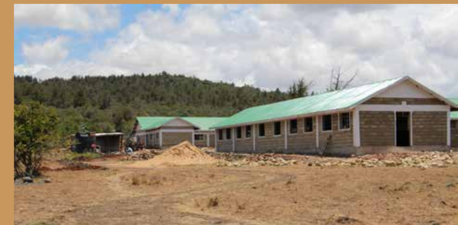
Ongoing construction at Lokusero to build the first secondary school in the area. Upon completion, the total number of the Lewa-sponsored schools will increase to 19.
